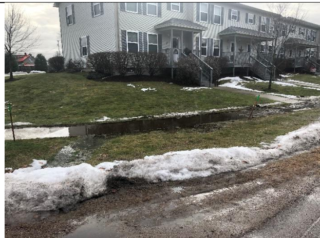
Photo 2: Runoff ponding on sidewalk along Checkerberry.
