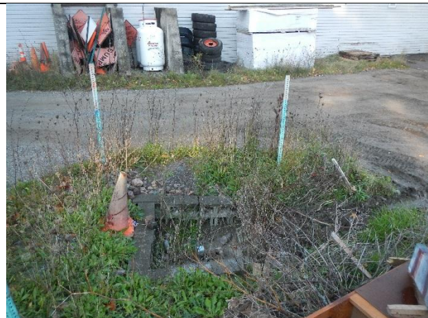
Photo 2: Deep catch basin with erosion
