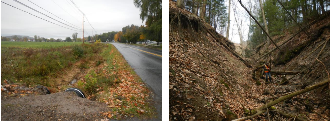
Figure 3: Two sites had the highest score (36 out of 50). Project O-1 (left) is located along North Rd where a large agricultural drainage flows to a roadside ditch with areas of erosion. The size of the drainage area and erosion along flowpaths into the ditch yield the highest estimated phosphorus load of all projects. Project SS-1 (right) is located on Stacy Street where a roadway drainage network is piped to a very large and active gully.
