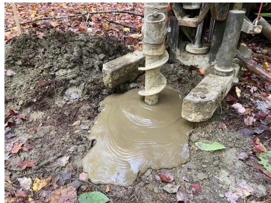
B-8 after boring collapsed
