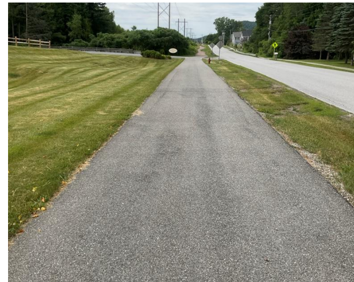
Photo 10: Typical paved sidewalk condition on Stacy Street
