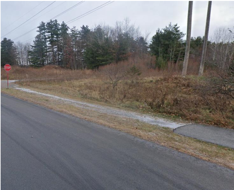
Photo 11: Paved asphalt sidewalk gap at Strawberry Lane
