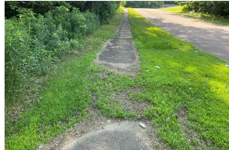
Photo 12: Typical vegetation overgrowth observed (very poor condition)
